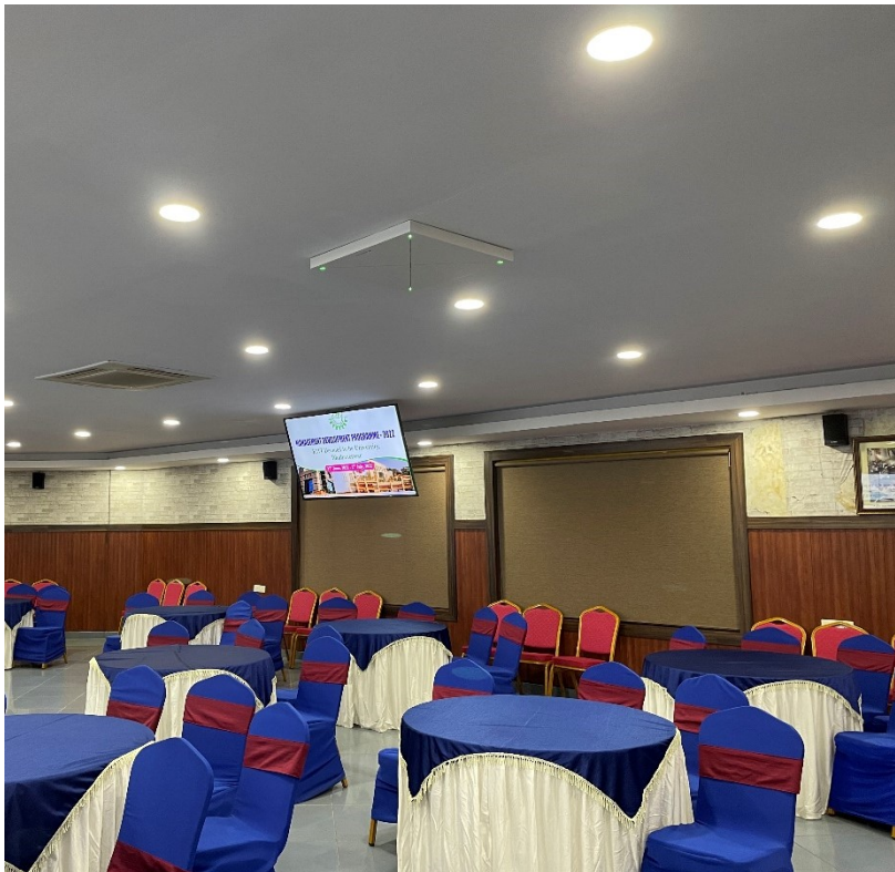
KIIT installed 150 units of Sennheiser TCC 2 to elevate the hybrid learning experience
